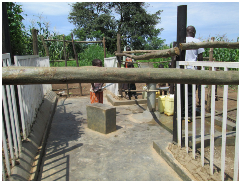
Some protective handrails and boreholes seats are not wellpositioned and act as a barriers to PWDs using tricycles
