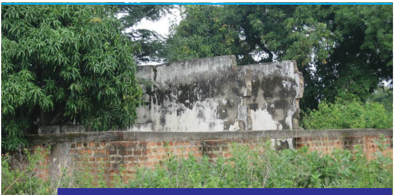
Ogor in Lira is one of the five Rehabilitation Centres that are no longer functional
